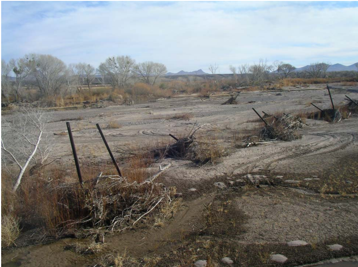
Photo 1. The bank and road protection facilities destroyed in the flood (wall constructed of 60-foot-long railroad rails, driven in place, and enclosed with flat bed railroad cars placed on end).
